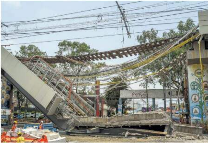
The section of the Mexico City metro that collapsed on May 3, sending a train plunging to the street and killing 26 people.
